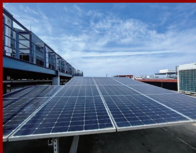
The rooftop photovoltaic system generates 800 MWh of green electricity to meet the energy demand of Lingang AIDC.
