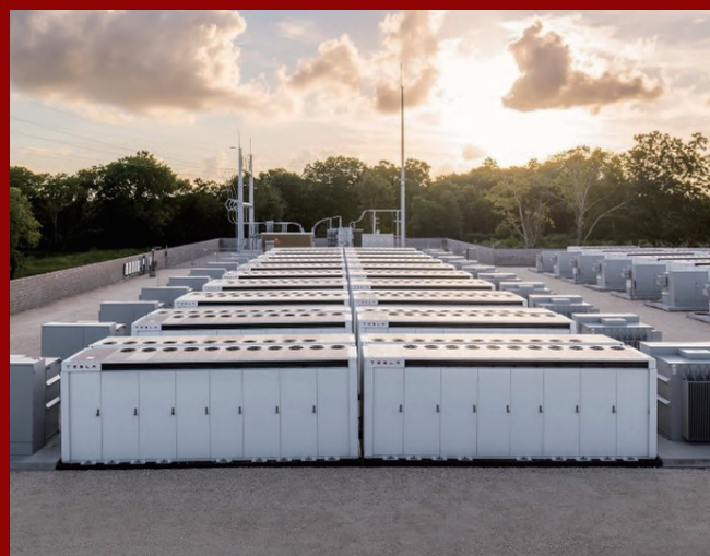
The integration of Tesla's Megapack system enables a smart and flexible power eco-system for Lingang AIDC.
